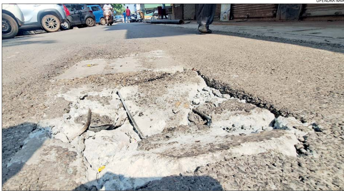
The damaged concrete drain cover with its metal bars exposed poses danger to motorists and pedestrians along the road near National Theatre, Panjim
